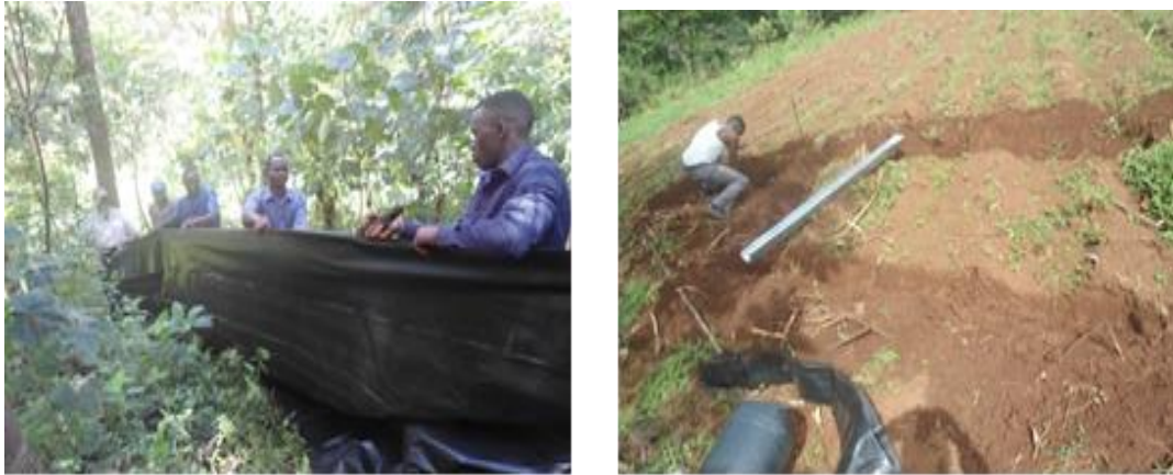
Figure 3.5: Pictorial view, Construction of Runoff Plots with the Help of the Community
