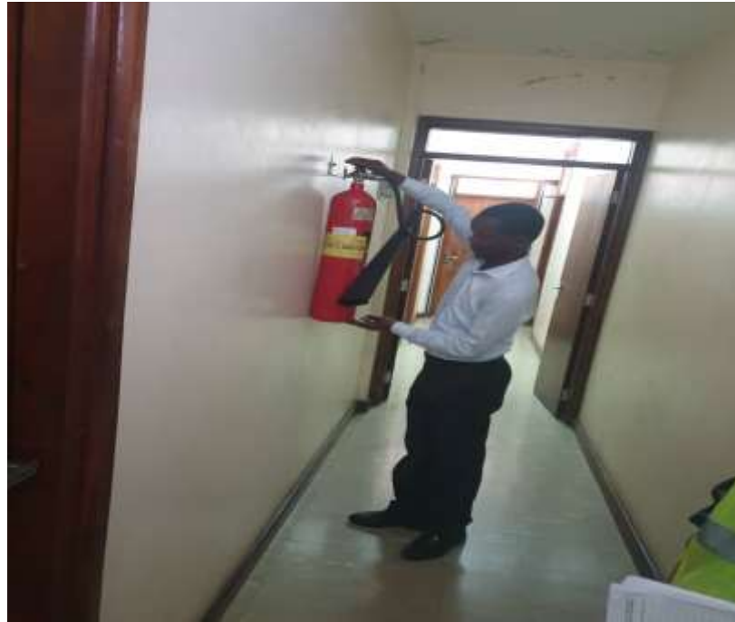
Plate 4.2: Portable Fire Extinguisher Mounted 120cm from the Floor (IA3)
