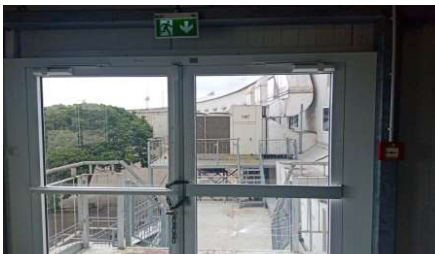
Plate 4.3: Locked and Chained Emergency Exit (IA1)
