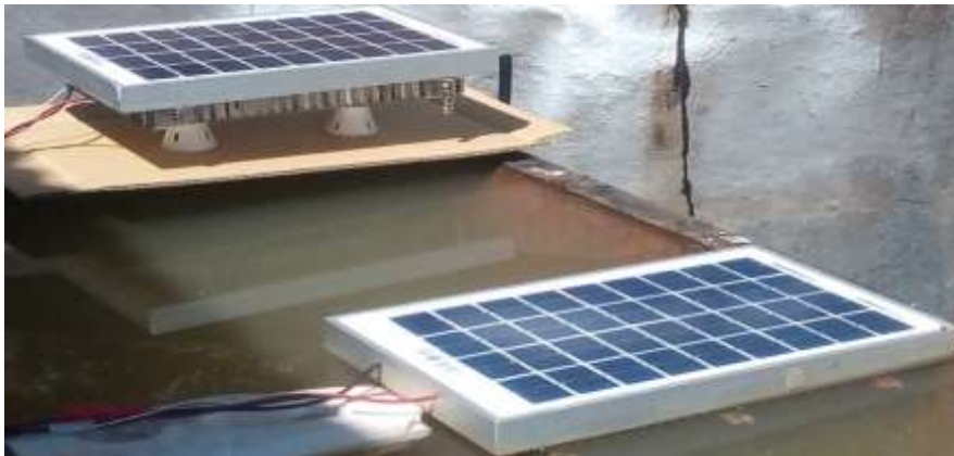
Figure 3.9: Battery Charging PV Temperature, Voltage and Current Measurement
