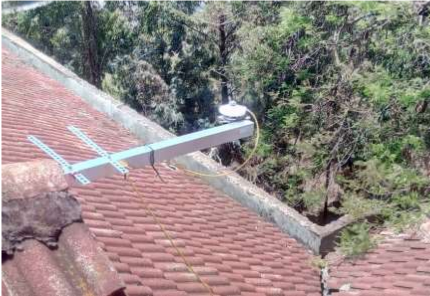
Figure 3.1: The CMP-3 Pyranometer on the IEET building roof
