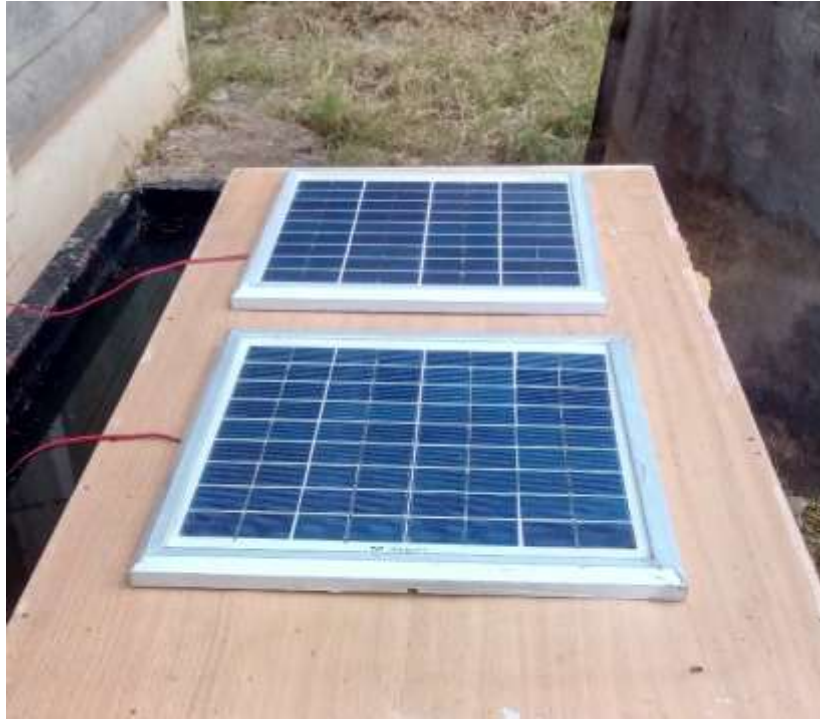
Figure 3.3: Characterization of the PV Modules
