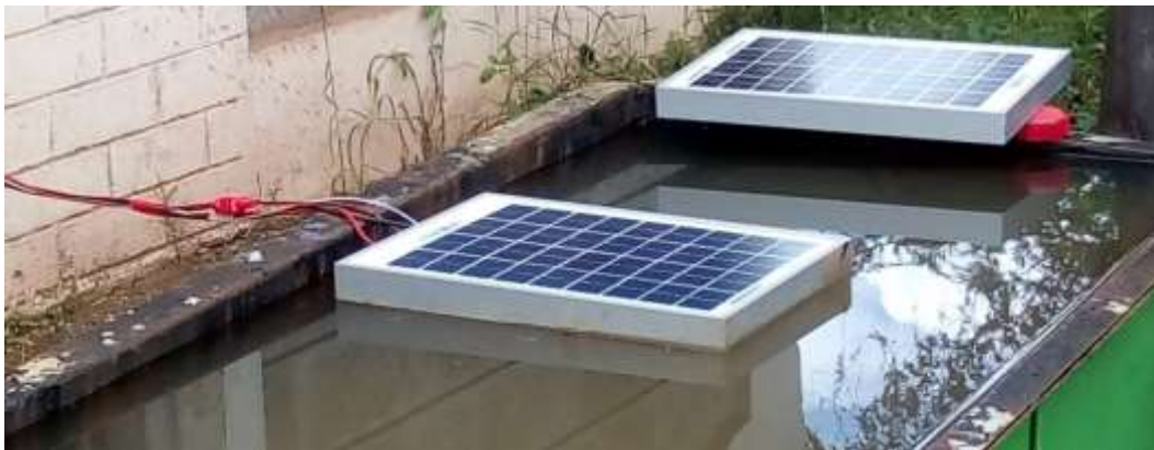
Figure 3.5: PV Module Temperature and Voltage Measurement
