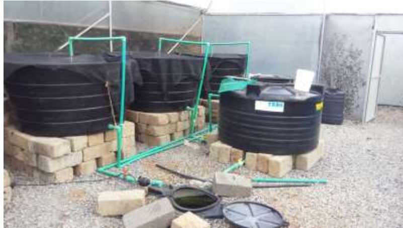
Plate F4: The RAS setup showing the production tanks, connection pipes, biofilter and sump tank
