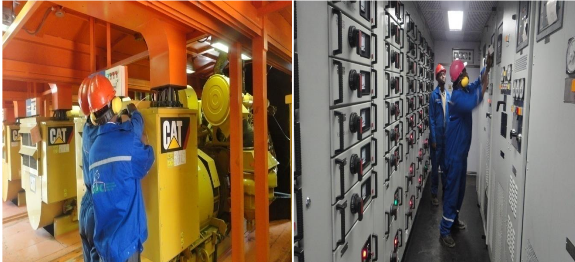
Plate 2.4: Inside the Generator Sets Room (left) and SCR Room (right) in a GDC Rig in Menengai (note the ear defenders)
