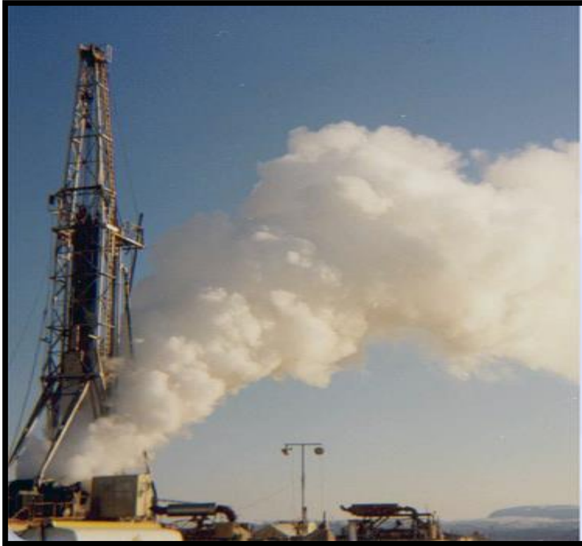
Plate 2.1: A blow out on a geothermal drill rig
