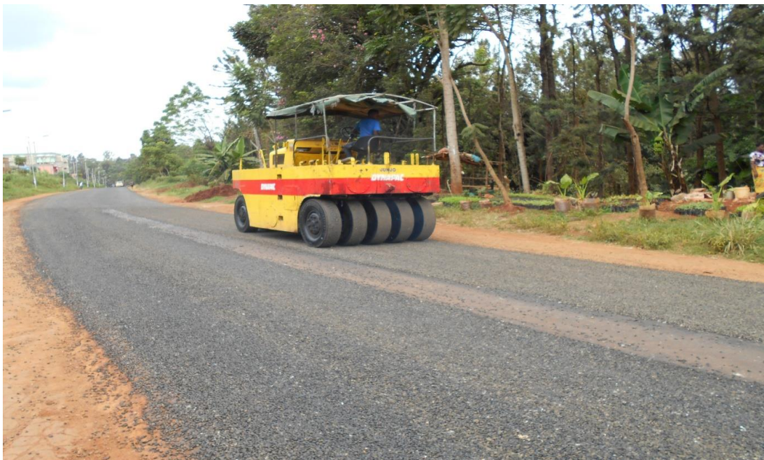
Plate 4.2: On going surface dressing on King'ong'o – Kiganjo road. No traffic cones or flagmen present on site
