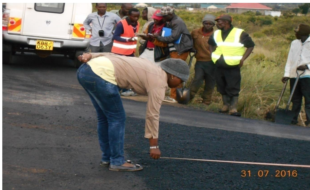
Plate 4.3: Measurements being taken by workers oblivious of the Physical and Chemical risks they are exposed to on Nyeri – Wiyumiririe road
