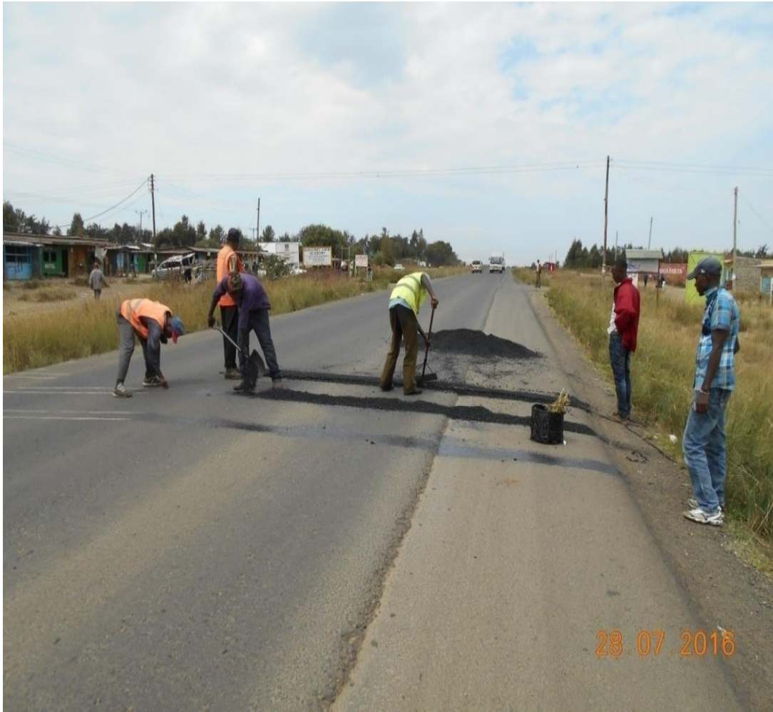
Plate 4.4: Installation of rubble strips on Marua -Karishen road. No safety cones and signage to protect workers from moving traffic
