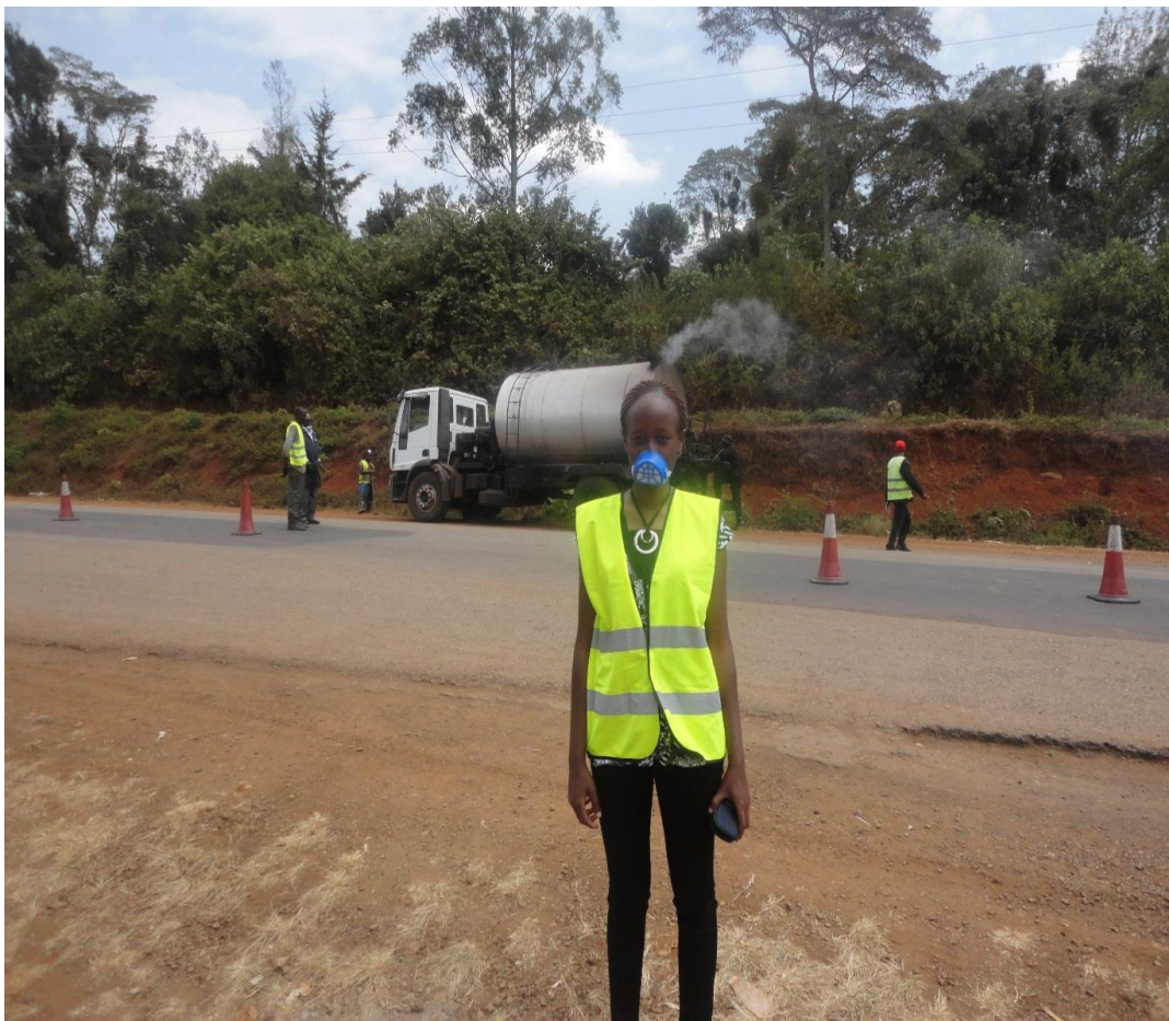
Plate 4.7: Dust mask provided to protect from inhalation of fumes from the bitumen road tanker on King’ong’o – Kiganjo road
