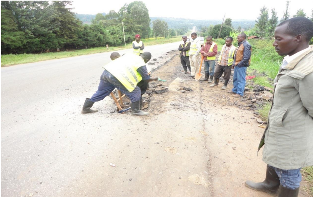
Plate 4.5: Workers on site on Sagana – Marua road. No safety cones and safety signage to protect the working area
