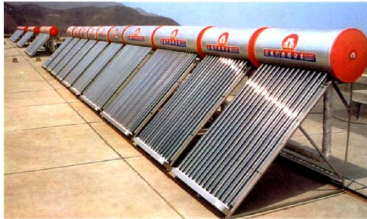
Figure 2.3: Evacuated Tube Solar Water Heater on roof top in China [54]
