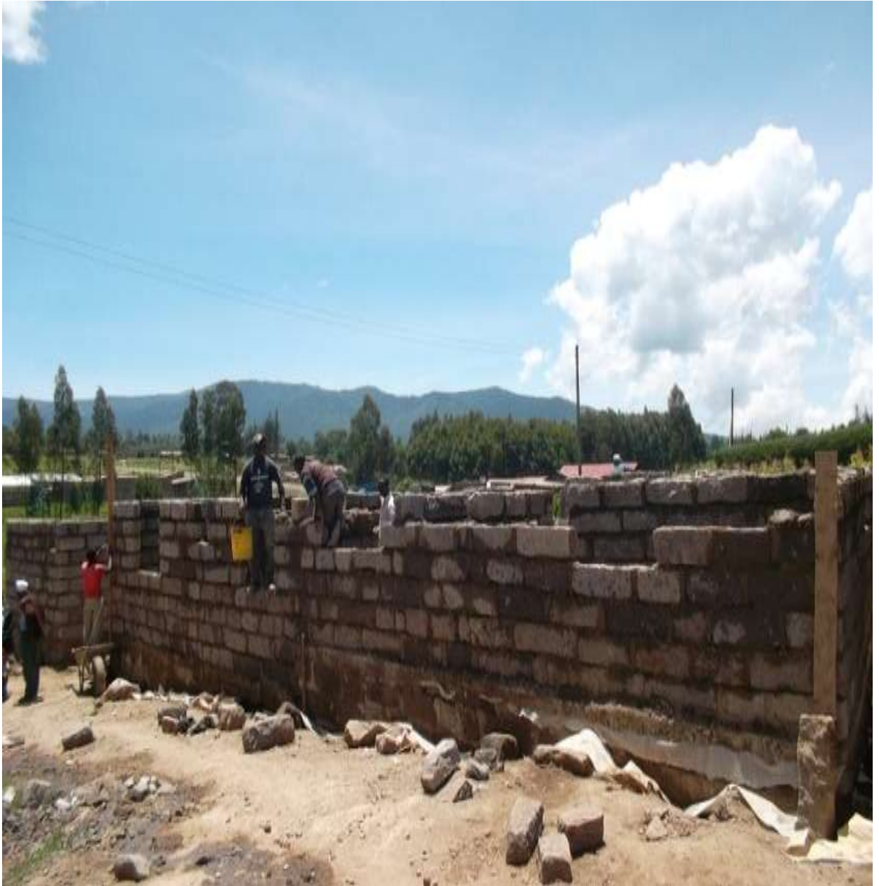
Plate 2: Working at height with no scaffold in Gilgil
