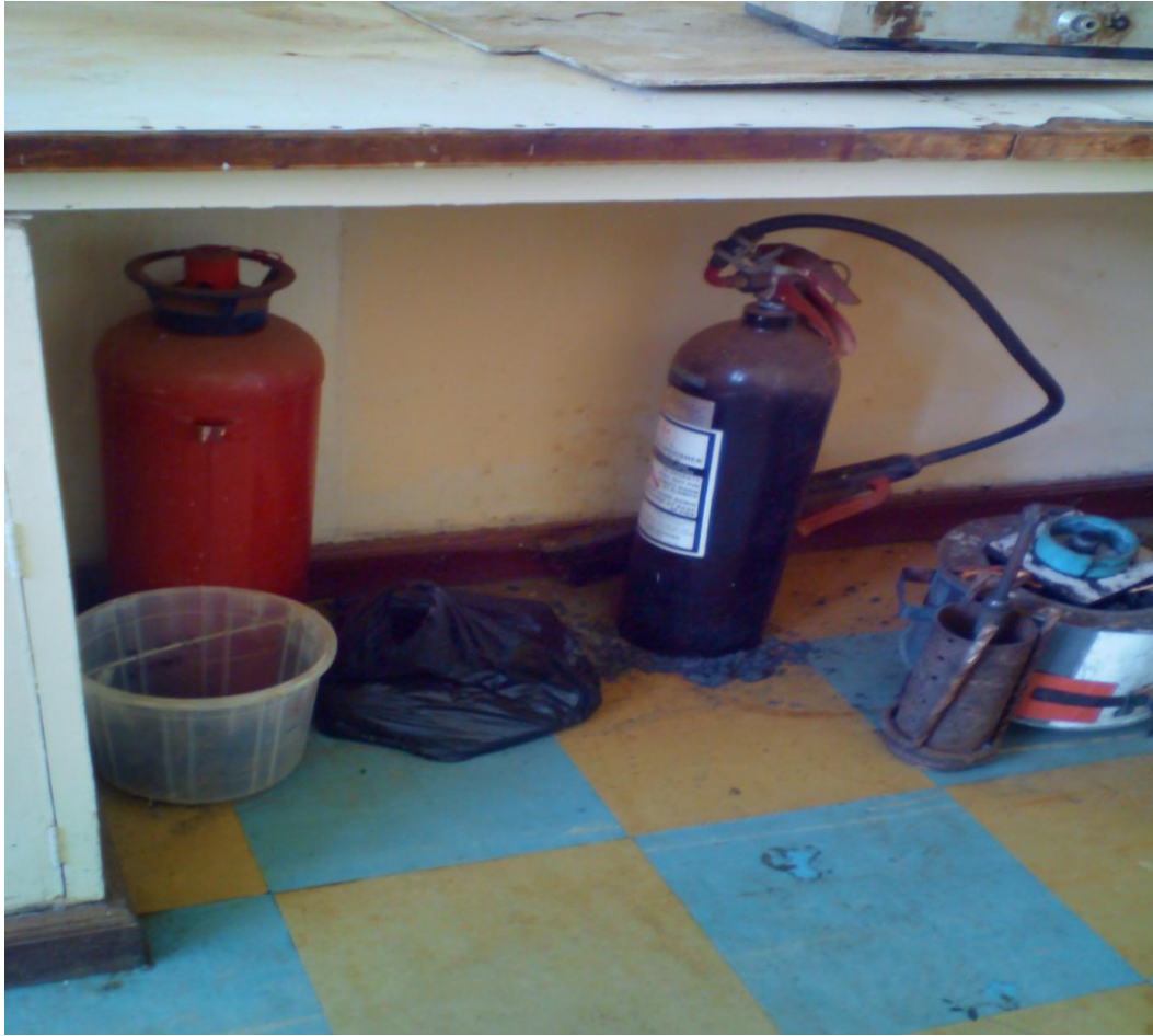
Plate 5: Improper placement of fire Extinguishers
