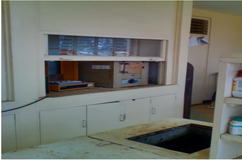
Figure 4. 5: Improper usage of fume hood chambers
