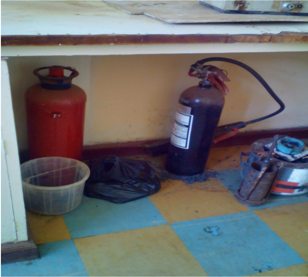
Plate 5: Improper placement of fire Extinguishers
