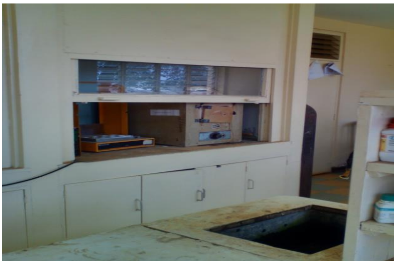
Figure 4. 5: Improper usage of fume hood chambers
