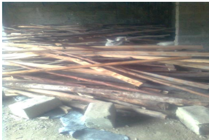
Plate 4.3 Formwork timber poorly stored on site.
