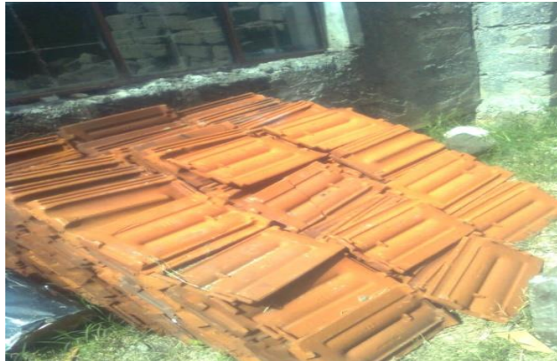
Plate 4.2. Roof tiles poorly stored cause for breakage.
