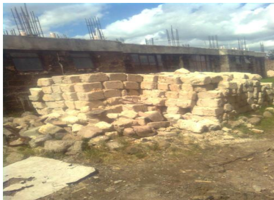
Plate 4.1. Sub- quality stones weathering out in the open. Source:
