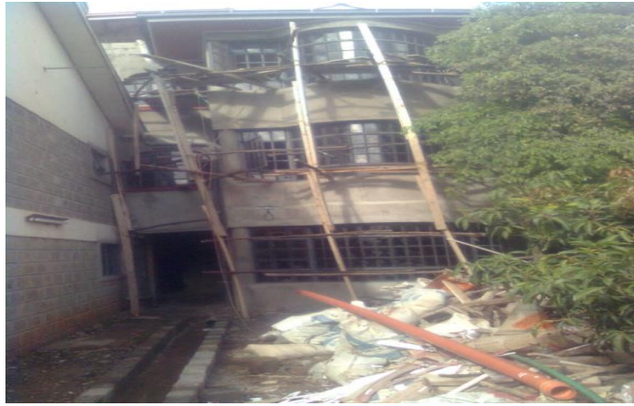
Plate 4.4 Mortar, concrete rubble dumped on site in cement bags for disposal
