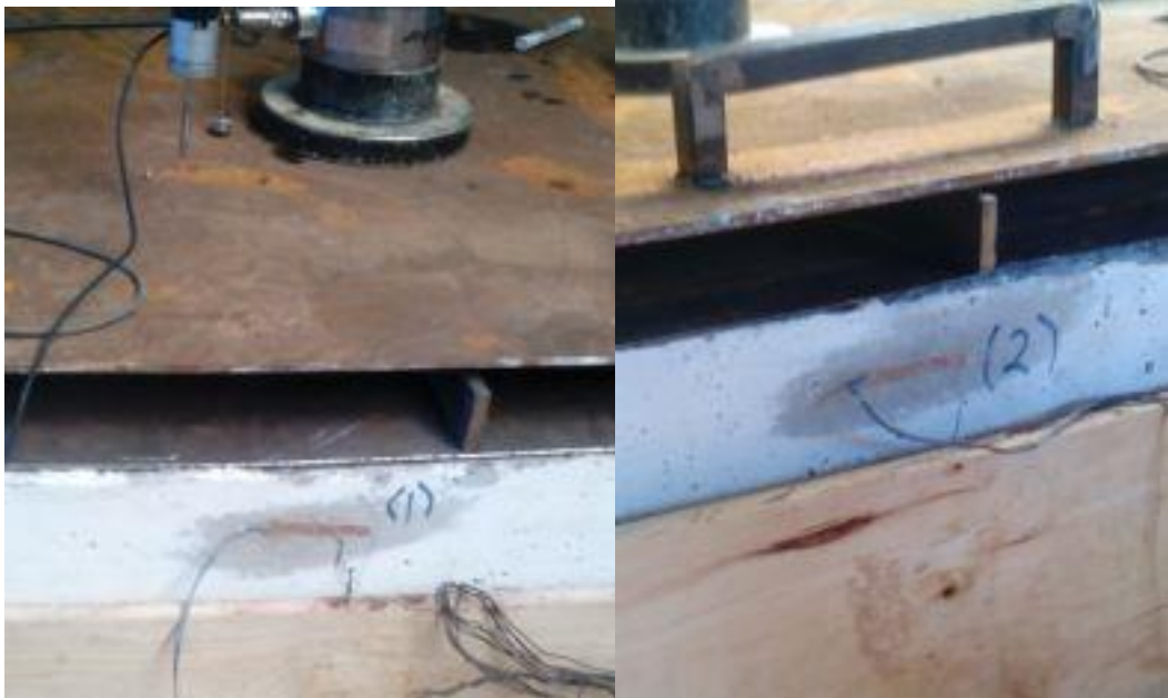
Plate 3.2: Failure Mode on All Four Faces is illustrated on Face 1 and 2
