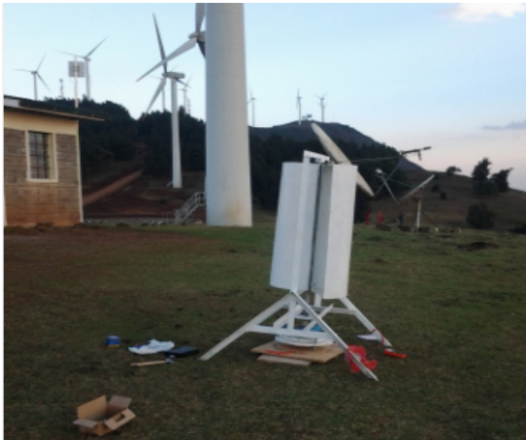
Plate 3.11: Rotor blade connected to a direct drive generator at Ngong' wind farm
