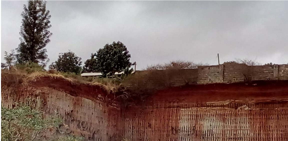
Figure 8: The picture shows the proximity of a homestead to an abandoned quarry that is not protected. The picture was taken during the survey
