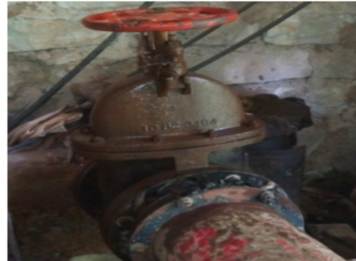
(b) Manually operated water flow control valve
