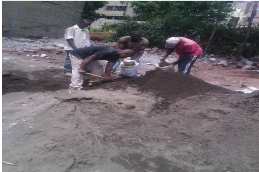
Plate 4.4: Employees working without PPE's (site 4)
