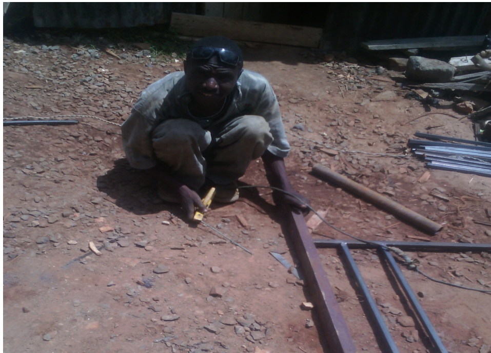
Plate 4.3: A worker with goggles but not utilizing properly (Site 1)
