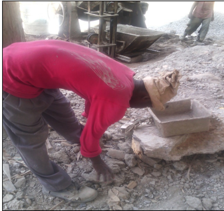
Plate 4.2: Workers using improvised PPE at construction sites (site 13)
