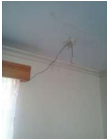
Internal air temperature and humidity sensor attached to ceiling in Thogoto house
