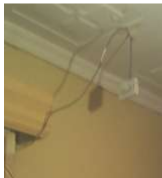
Internal air temperature and humidity sensor attached to ceiling in Syokimauhouse
