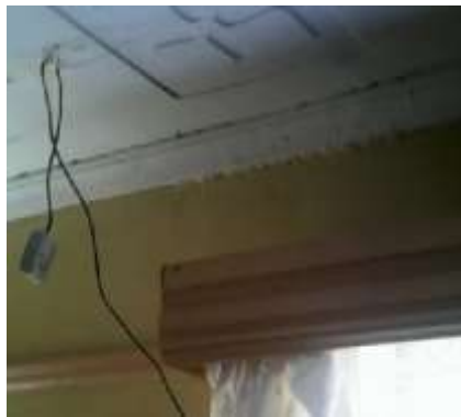
Internal air temperature and humidity sensor attached to ceiling in Dandorahouse
