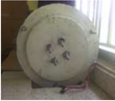
Plate 3.26: Generator front view
