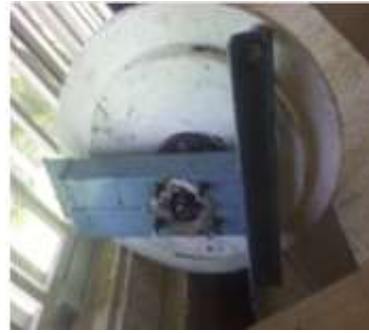
Plate 3.27: Generator back view
