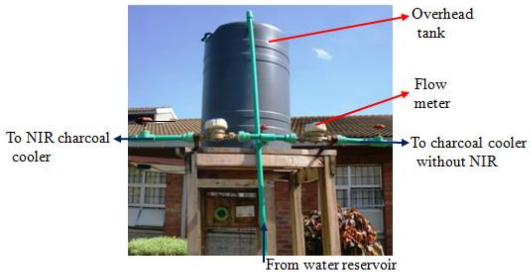
Figure B5 A photograph of the water distribution system for both the S_{NR} and S_{NNR}
