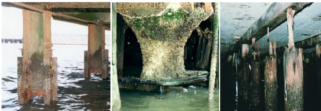
a) Corroded steel piles b) Degraded concrete pile c) Deteriorated timber piles Plate 1.1 Degradation of conventional piles [6]
