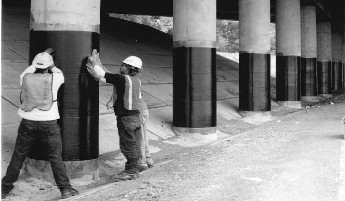
Plate 2.1 FRP wrap being installed on a highway column in California, USA (Courtesy of Sika Corporation)
