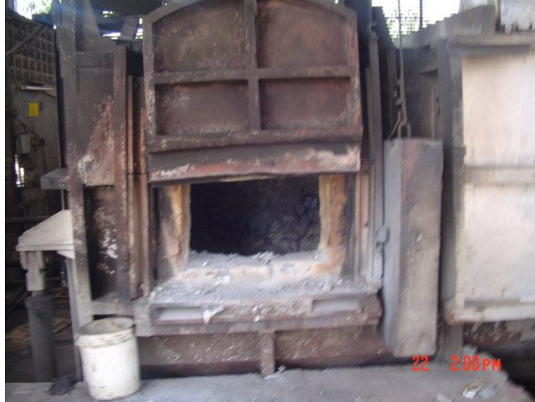
Figure 5.12: Furnace with no temperature control for melting aluminium scrap: Courtesy of Booth Extrusions Ltd, Thika
